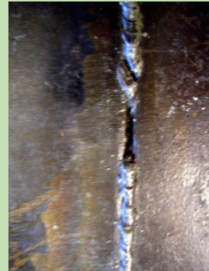
Incomplete root penetration
